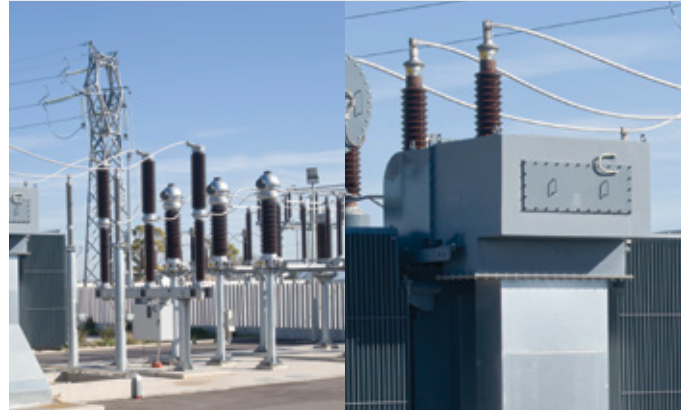
An LTC plays a critical part in a transformer's operation
