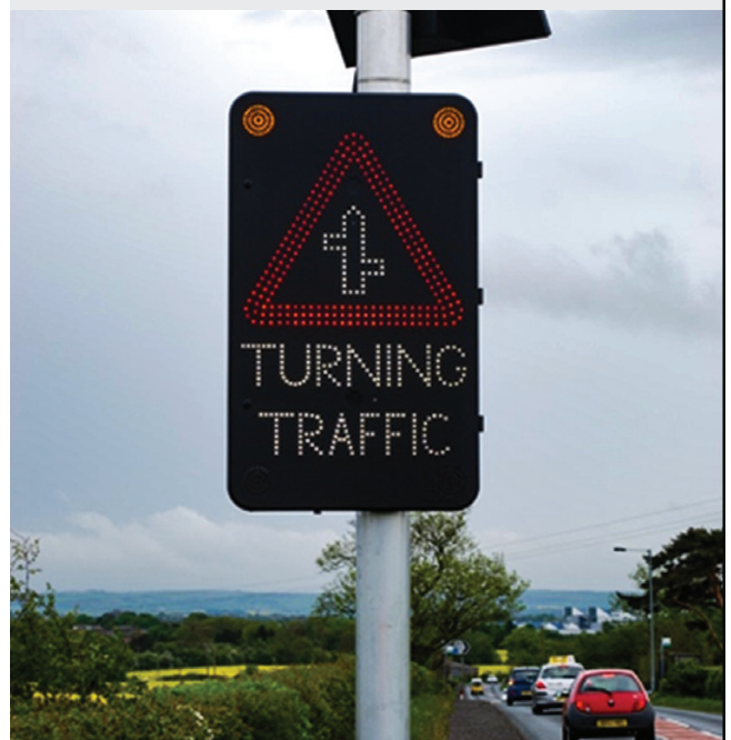
Upon detection by the FLIR TrafiOne, the electronic warning signs are activated.
