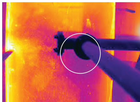
LD#2 caster- leakage through tundish heating line blanking joint.
