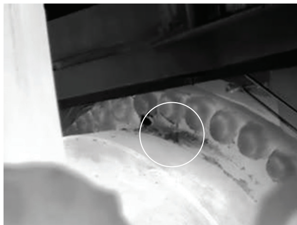
HBF leakage through GV #1
