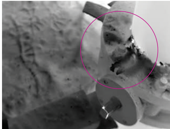
HSM pipe leakage at FCE #1
