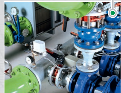
... pumps used in industrial plants
